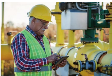
▲ Fuel supply inspection
